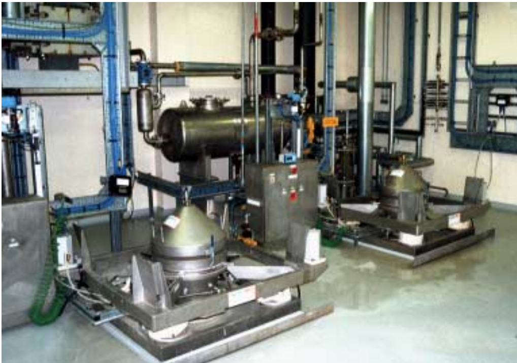
Gravimetric Discharge Stations
