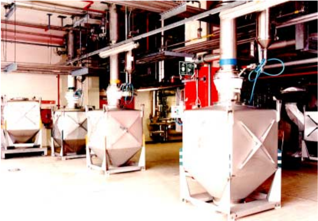
Manual Lift/Lower IBC Filling Heads in operation
